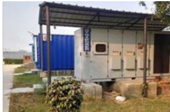
BESS at Central Electronics Ltd, Sahibabad by Newen
